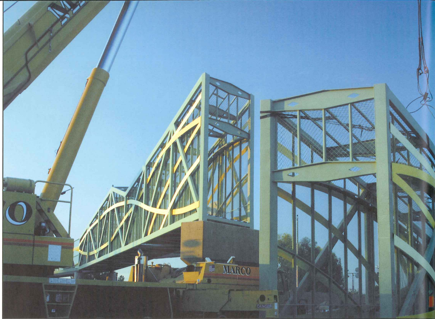
JUDY BALES Maryland Avenue Bicycle and Pedestrian Bridge . Installation process in 2005. Steel, concrete, metal mesh. Artist collaboration with engineer Jerry Cannon for design of superstructure, ramps, and landscaping for steel truss bridge, 25' x 250' x 10', 2005. Photo: Richard Strange. RIGHT: JUDY BALES Maryland Avenue Bicycle and Pedestrian Bridge . Interior view.
